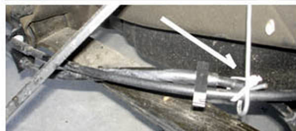
elevate and secure cables
